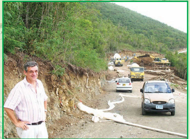
Jan vanden Eynde of ICE looks on at the progress being made on the roads and drainage system for phase 2 of the Valley Estates project.
